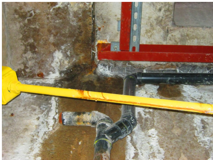
Figure 9 Active leaks observed around the access hatch to the electrical room (looking up)
