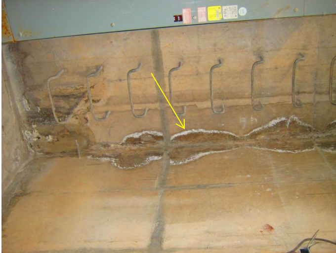
Figure 10 Signs of non-active leaks observed at the corner wall of the electrical room (photo rotated 90 degrees clockwise)
