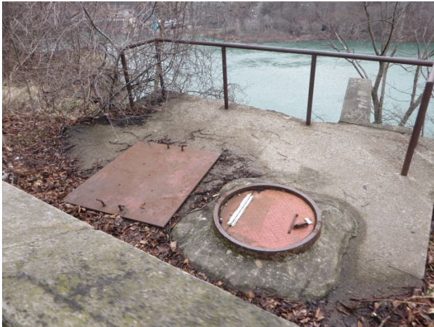
Figure 12 Unsecured access hatch and inadequate railing around the exterior drop shaft to the Niagara gorge
