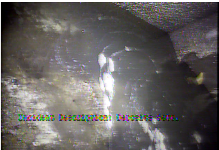
DSGV - Deposits Settled: Gravel @ 0.0 m.
