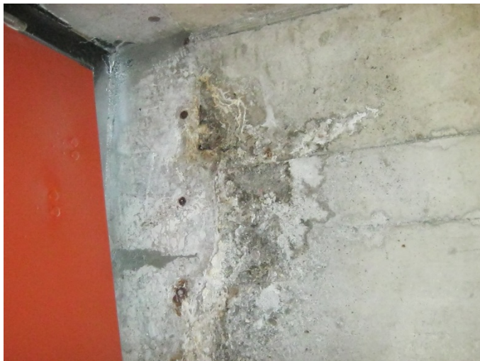
Figure 6 Honeycombing and exposed rebar at the interface between the original and new dry well structures (looking up, outside electrical room door)
