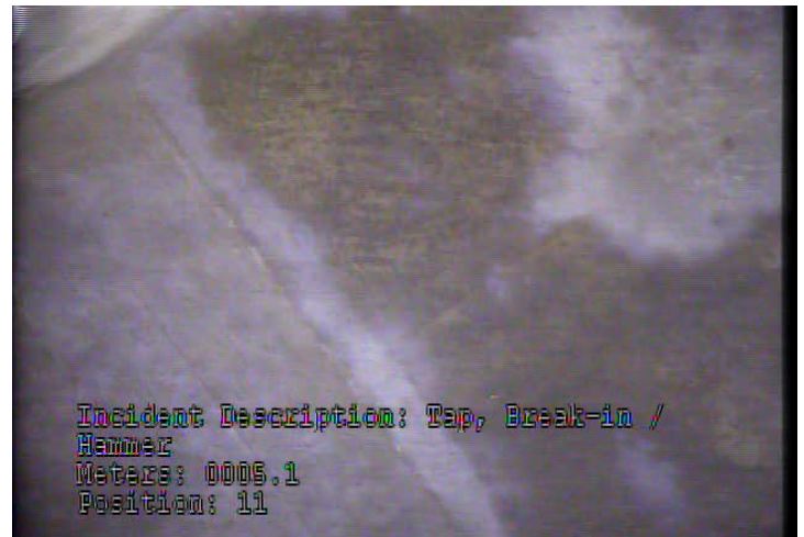
TB - Tap, Break-in / Hammer @ 5.1 m.
