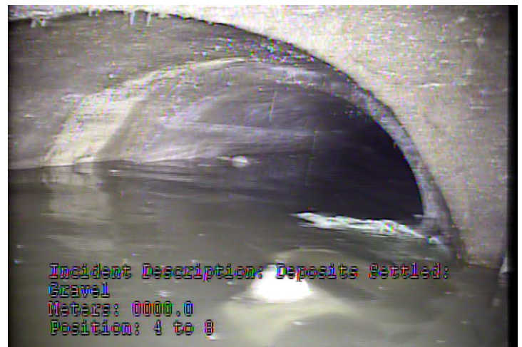
DSGV - Deposits Settled: Gravel @ 0.0 m.
