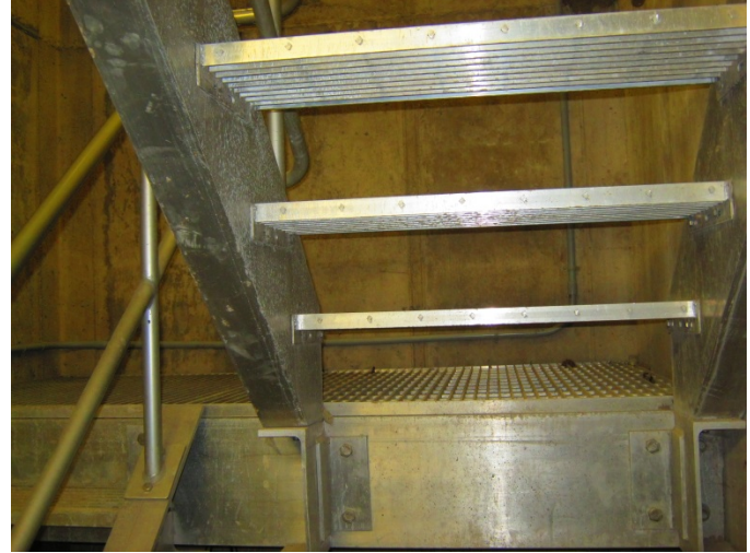
Figure 11 Existing staircase in the dry well was found to be in good shape. However, additional supports are recommended for the railings.
