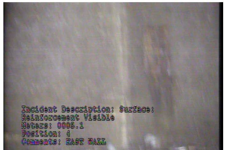
SRV - Surface: Reinforcement Visible @ 5.1 m. EAST WALL
