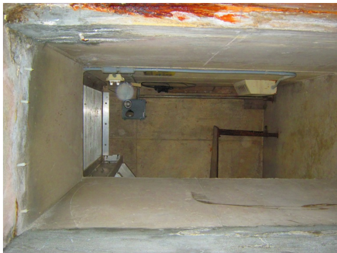
Figure 7 Signs of cracks and failed polyurethane injections at the interface between the original and new dry well structures (dry well lower level, looking towards the staircase, photo rotated 90 degrees counterclockwise)
