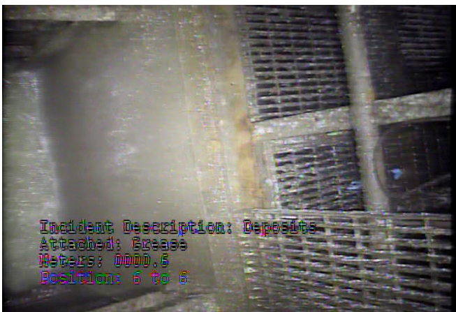
DAGS - Deposits Attached: Grease @ 0.6 m. COVERING MOST OF LOWER CHAMBER
