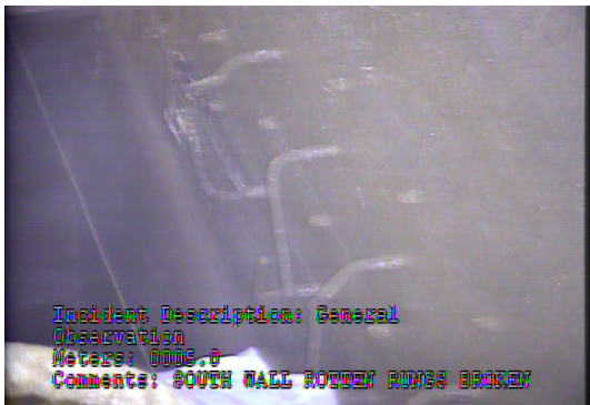
MGO - General Observation @ 5.0 m. SOUTH WALL ROTTEN RUNGS BROKEN NO H2S ATTACK ON SOUTH WALL REBAR AT BOTTOM BY FLOOR GRATING
