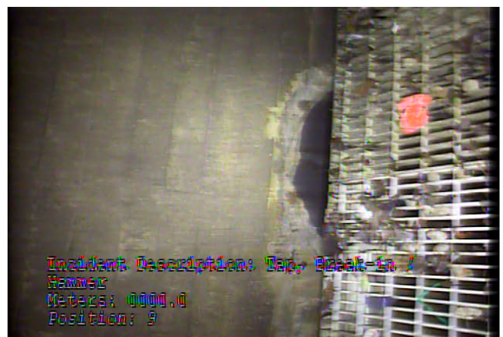
TB - Tap, Break-in / Hammer @ 0.0 m.
