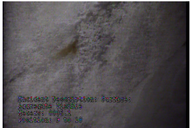
SAV - Surface: Aggregate Visible @ 5.1 m. NORTH WALL
