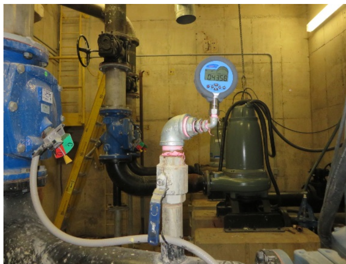
Figure 2 High resolution pressure logger mounted at the pump discharge
