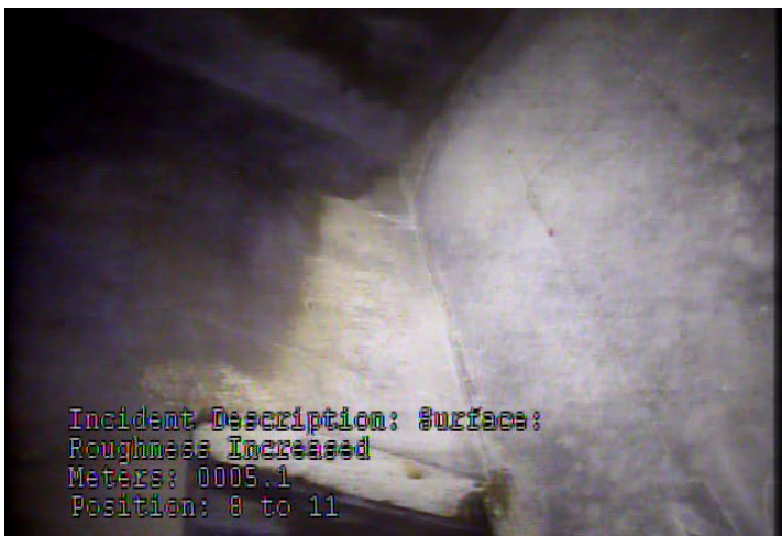
SRI - Surface: Roughness Increased @ 5.1 m. WEST WALL ABOVE DOOR
