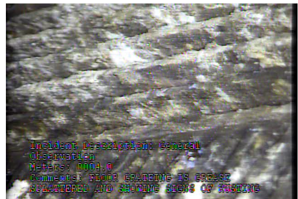
MGO - General Observation @ 4.0 m. FLOOR GRATEING IS GREASE SPLATTERED AND SHOWING SIGNS OF RUSTING
