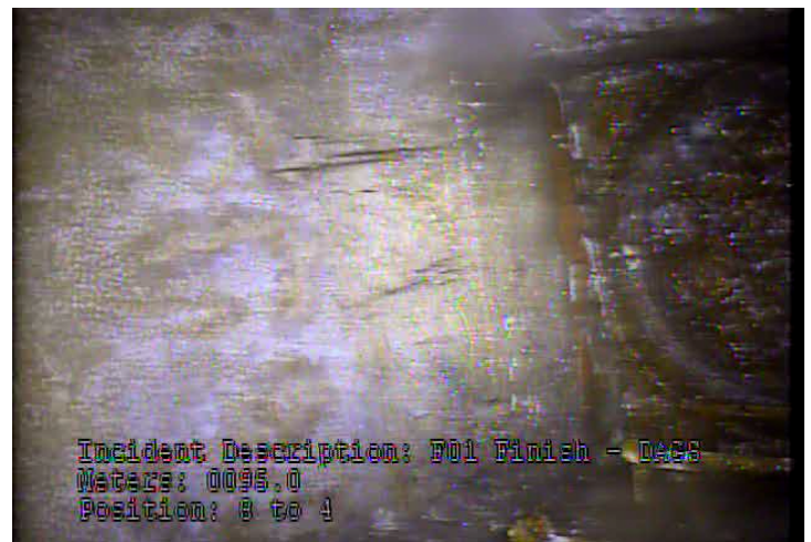
DAGS - Deposits Attached: Grease @ 95.0 m.
