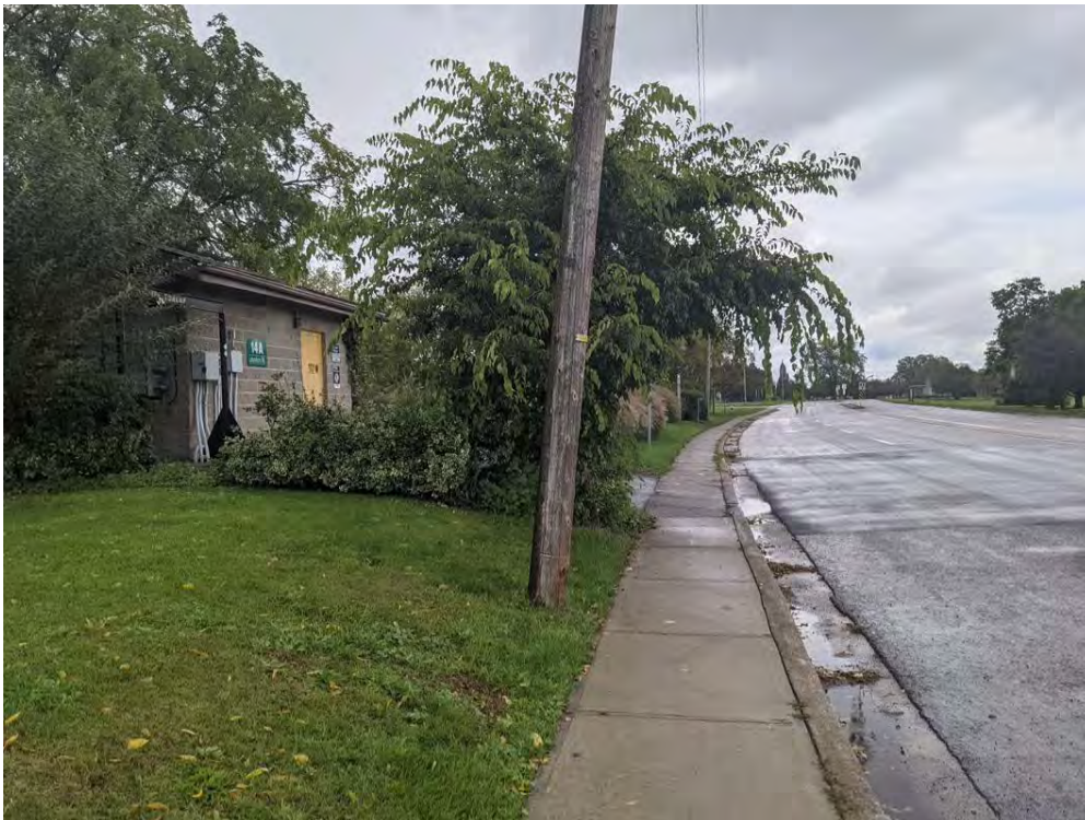
Image 10: View of Lakeshore Road SPS structure, exhibiting extensive disturbance, facing north
