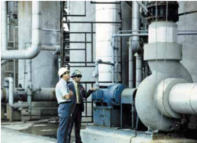
A 3175 installed in a major chemical plant.
