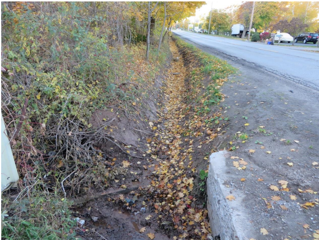
Photo 12: Example of conditions surrounding tributary to Konkle Creek east of 5366 King Street.
