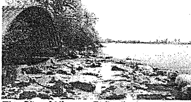
The City of Niagara Falls discharged sewage into the upper Niagara River, a little more than a kilometre upstream of the intake to the city's water treatment plant, from this storm culvert in heavy rains in December
