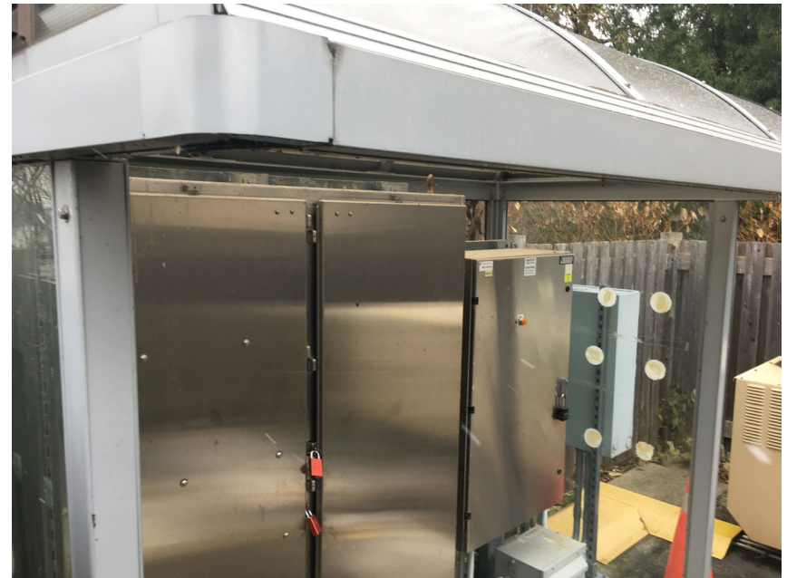
Example Shelter for Electrical Panel
