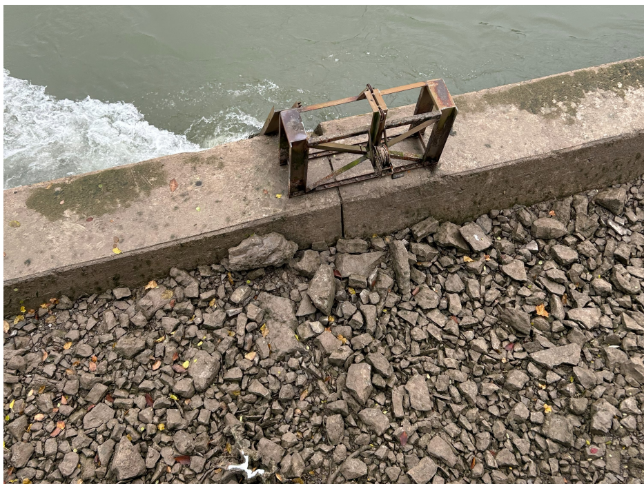
Figure 39: Existing Gate Valve
