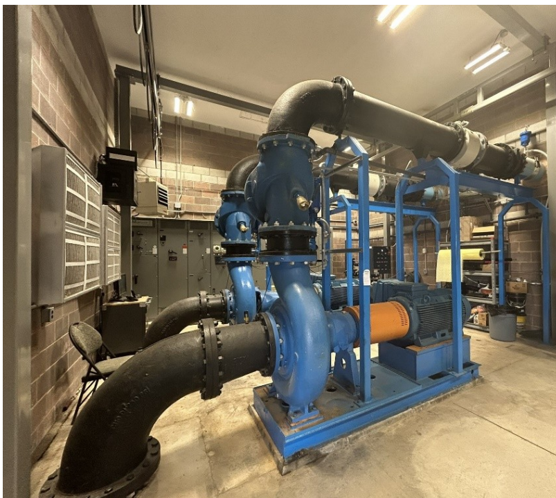
Figure 32: Existing Pumps at Dee Road Pump Station
