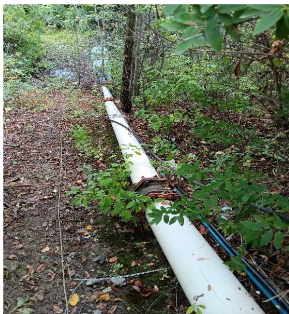
Figure 48: Existing 200-millimetre Pipe
