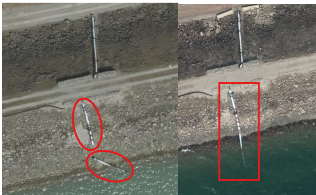
Figure 27: Destroyed Siphon 2013 and Repaired Siphon 2018
