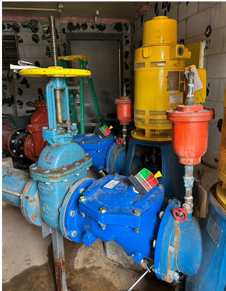
Figure 37: Existing Pumps at Whirlpool Pump Station
