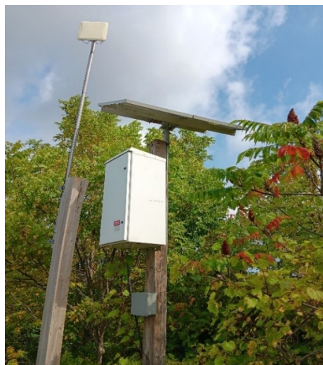
Figure 52: Solar Panel–Supplied Electrical System for the Flowmeter
