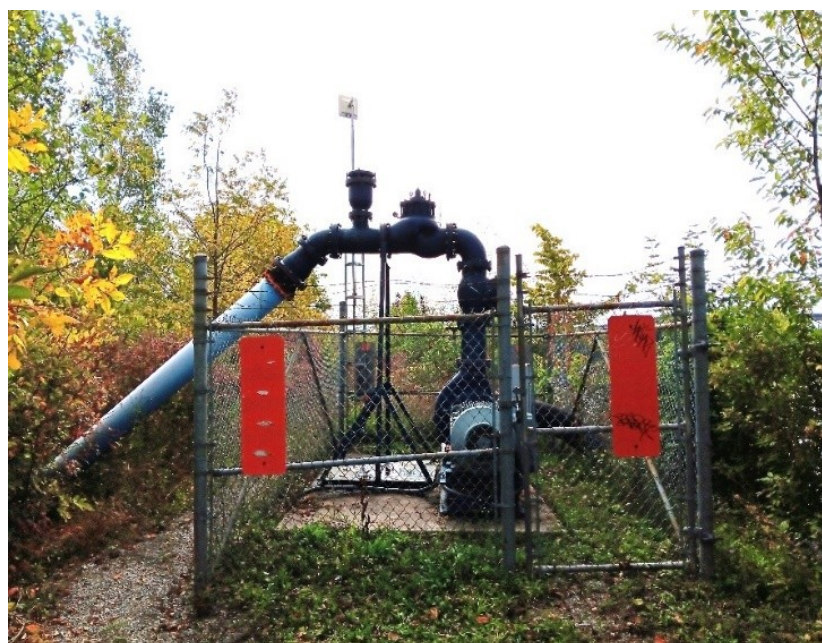
Figure 43: Existing Self-priming Pump at Eastchester
