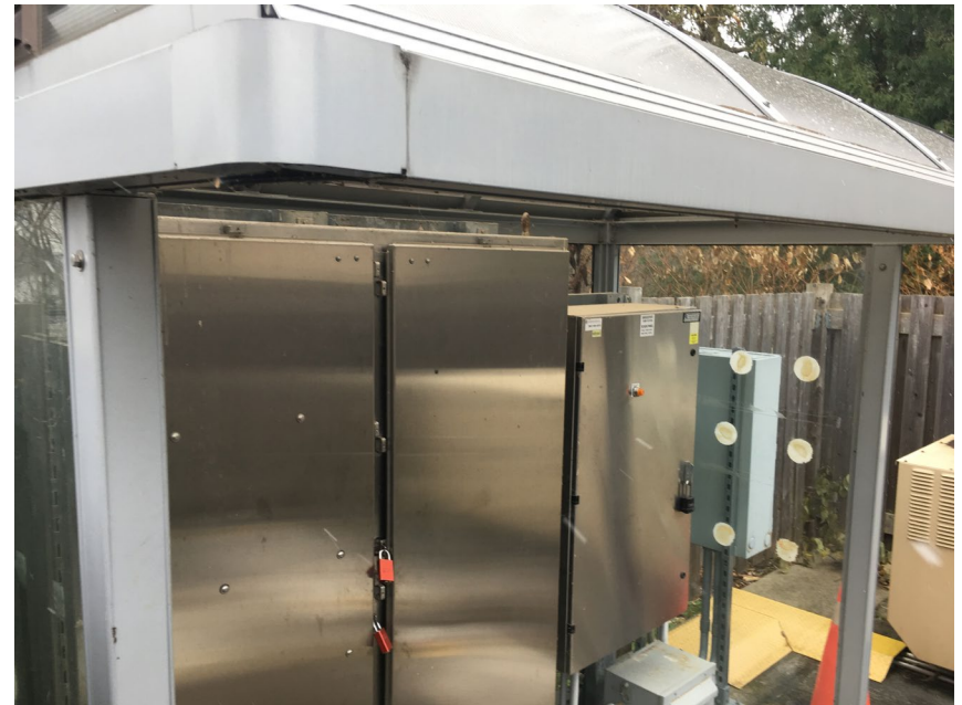
Example Shelter for Electrical Panel
