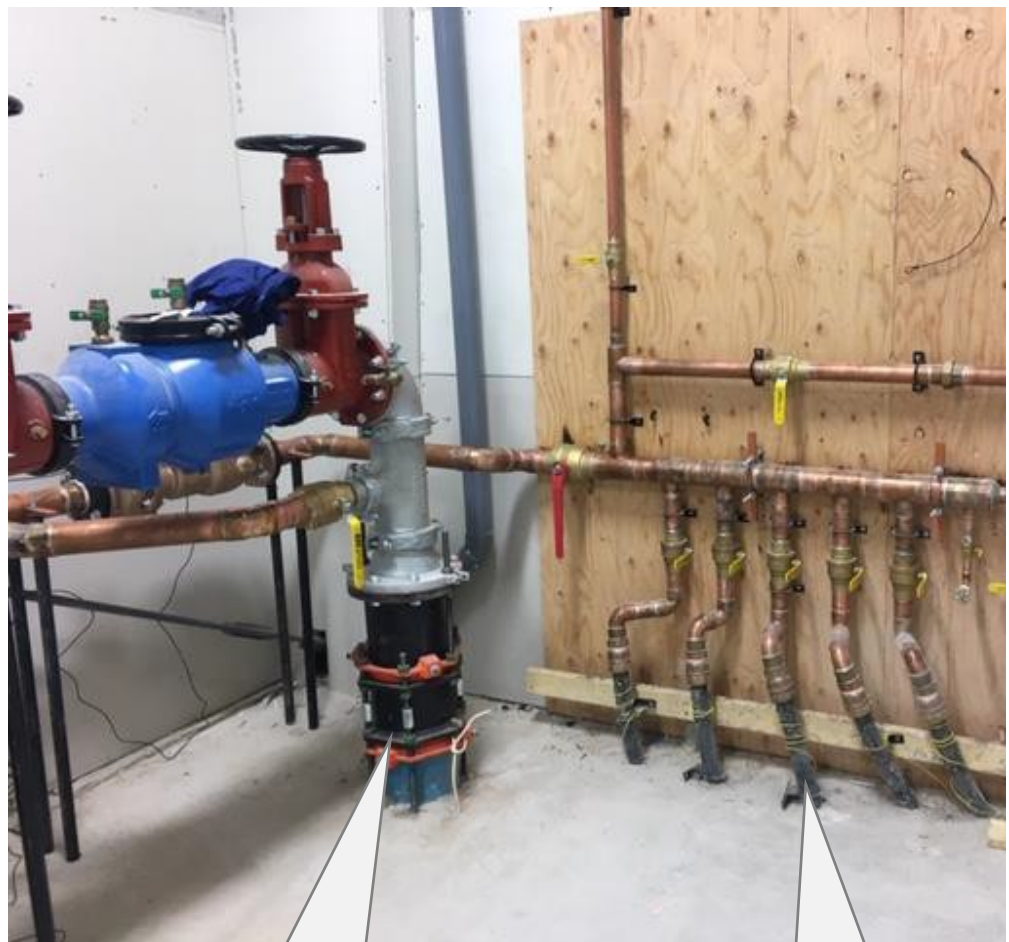
Incoming water service measurement point
