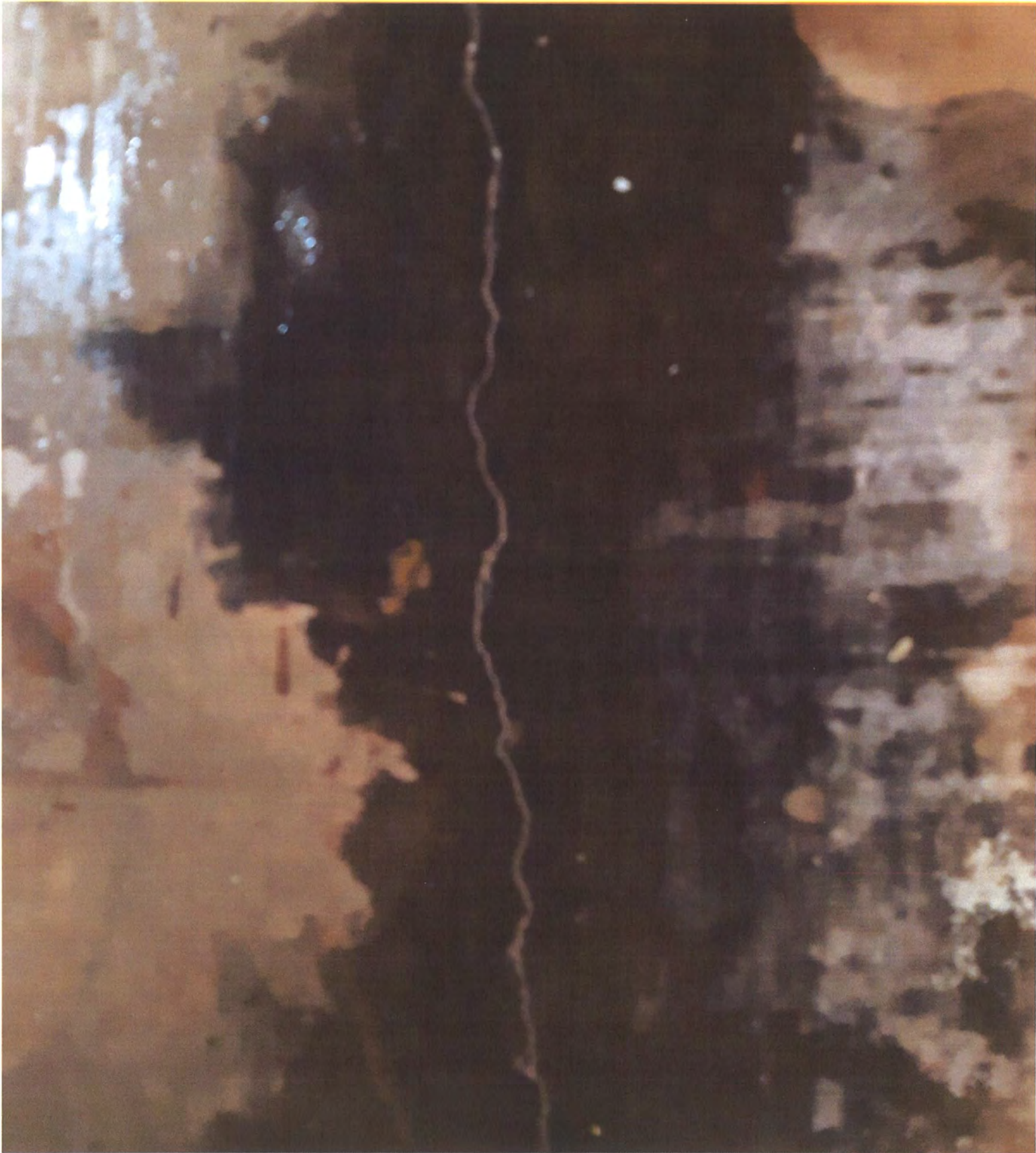
Crack in basement floor
