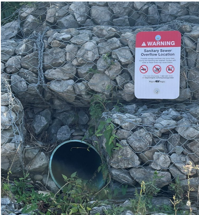
Figure SW-C- 2 - Image of Sanitary Sewer Overflow Public Signage
