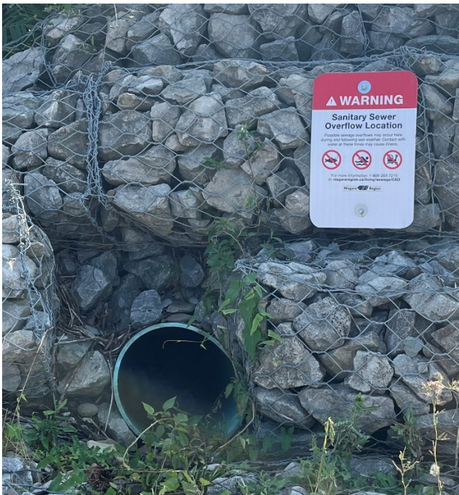
Figure PW-C- 2 - Image of Sanitary Sewer Overflow Public Signage
