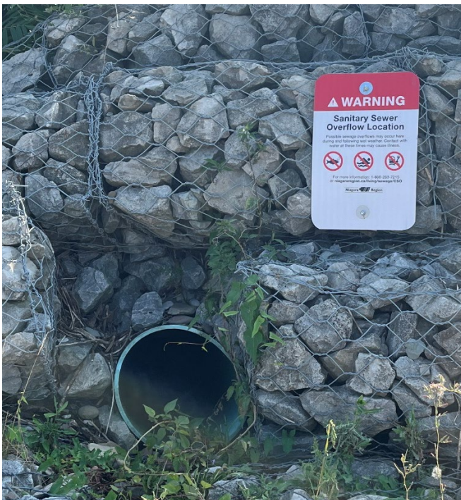
Figure PD-C- 2 - Image of Sanitary Sewer Overflow Public Signage
