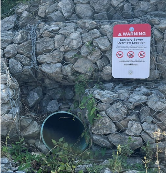
Figure CB-C- 2 - Image of Sanitary Sewer Overflow Public Signage
