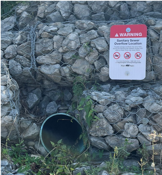
Figure BR-C- 2 - Image of Sanitary Sewer Overflow Public Signage
