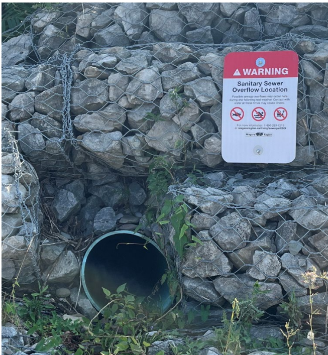
Figure AA-C- 2 - Image of Sanitary Sewer Overflow Public Signage
