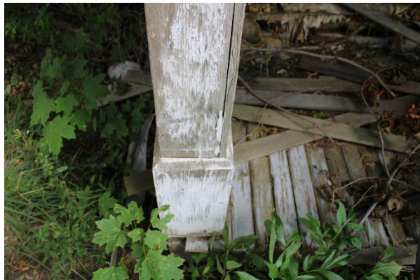
Plate 44: Example of wood footing on a pillar supporting the veranda roof on the south elevation.
