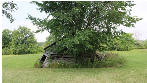
Plate 84: Collapsed Outbuilding 2, east elevation
