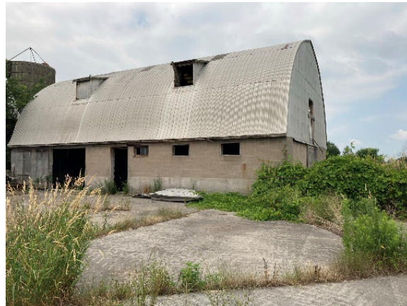
Plate 90: Barn 2 with concrete foundations/blocks and gothic arch aluminium roof, east and north elevations
