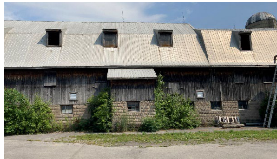
Plate 68: Barn 1 with vertical board upper siding, rusticate concrete block foundations, and shed style dormers, facing north
