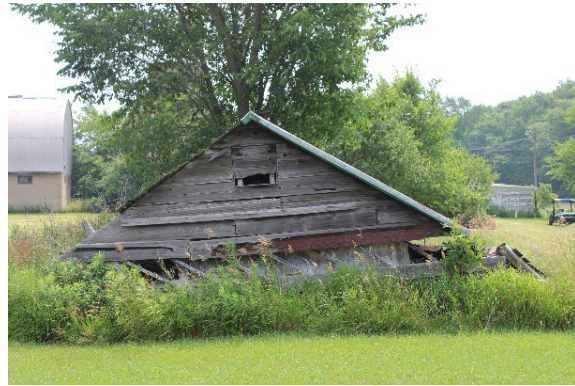
Plate 82: Collapsed Outbuilding 2, west elevation
