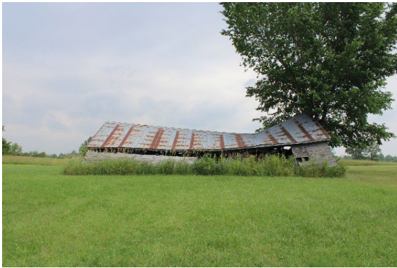
Plate 81: Collapsed Outbuilding 2, south elevation
