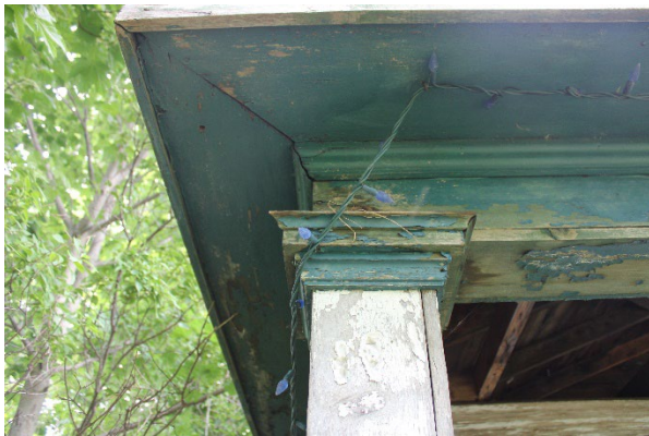
Plate 43: Moulded wood cap on the wood pillar supporting the veranda roof (south elevation)
