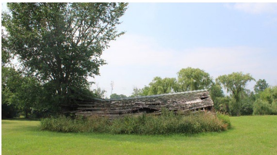
Plate 83: Collapsed Outbuilding 2, north elevation
