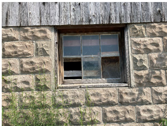
Plate 70: Example of wood frame, six light window located on lower level of Barn 1
