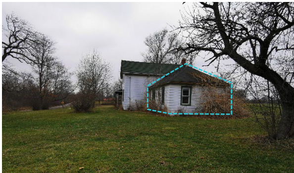
Plate 49: East elevation of 6811 Reixinger Road with Addition B outlined in blue hatching
